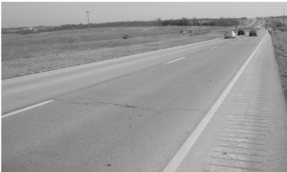
Figure 1. Reflective cracks on US36 near Cameron, MO.
