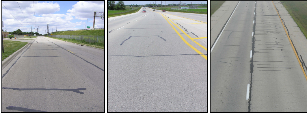
Figure 1. Thermal cracking in asphalt concrete pavements.
