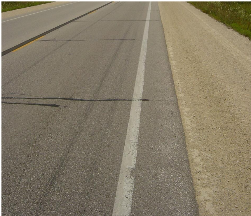
Figure 1-6: Thermal Cracking in Asphalt Pavement
