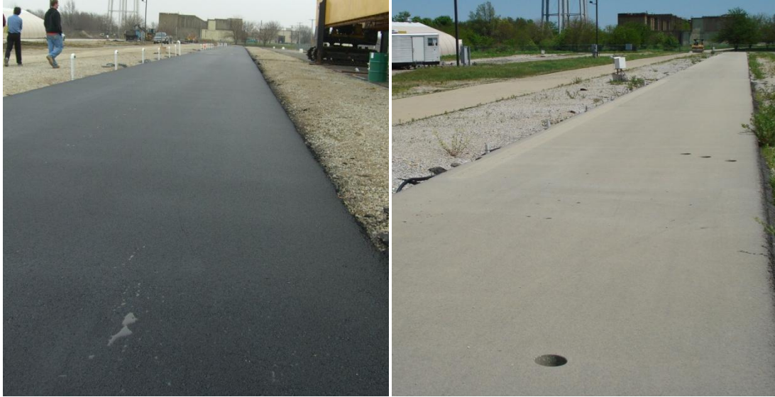
Figure 6-1: Pavement Section at ATREL (left: immediately after construction right: 19 months after construction)
