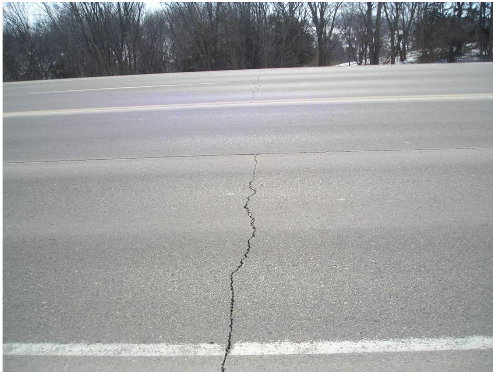
Figure 1-7: Reflective Cracking in Asphalt Overlay
